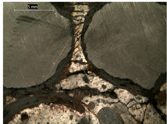
Stereo-optical micrograph of polished cross sectioned core showing corrosion and corrosion induced cracking of steel rebar.
