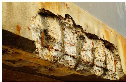
Corrosion damage on a concrete bridge on a busy thoroughfare in Frankfurt, aged about 50 years.
