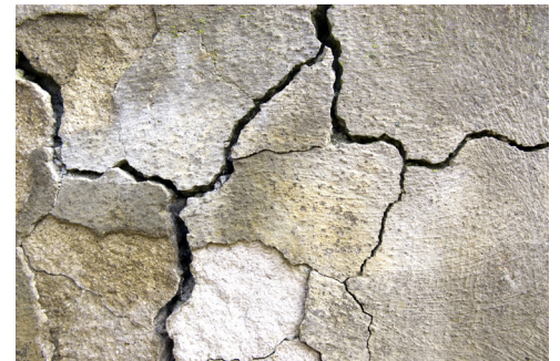
Figure 2. Cracked concrete foundation wall.
