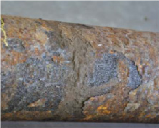
Figure: External pipe corrosion (RJLG photo)
