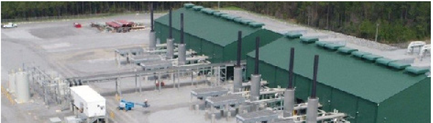
Figure: Natural gas compressor station
