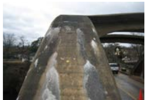
Figure 2. ASR-affected Bibb Graves Bridge in Wetumpka, Alabama, showing cracking and gel exudation features.
